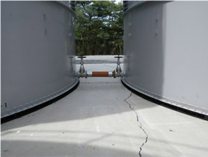
In this photo taken in July, 2011 and released Saturday, Aug. 24, 2013 by Tokyo Electric Power Co., a crack on the foundation concrete under a storage tank at the H1 area at the tsunami-crippled Fukushima Dai-ichi nuclear power plant in Okuma, Fukushima Prefecture, northeastern Japan, is shown. (AP Photo/Tokyo Electric Power Co.)
