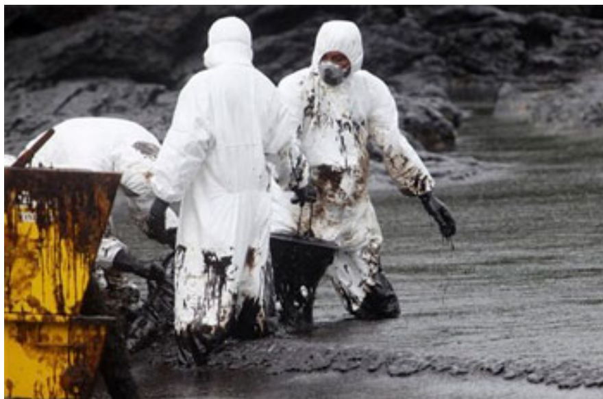
Workers remove crude oil during a clean up operation on the beach of Prao Bay on Samet Island in Rayong province eastern Thailand Tuesday, July 30, 2013. About 50,000 liters (13,200 gallons) of crude oil that leaked from a pipeline operated by PTT Global Chemical Plc. has reached the popular tourist island in Thailand's eastern sea despite continuous attempts to clean it up. (AP Photo)
