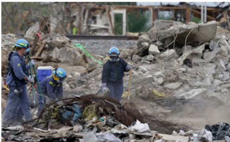
Investigators sift through the debris of the destroyed fertilizer plant in West, Texas, Thursday, May 2, 2013. Investigators face a slew of challenges in figuring out what caused the explosion at the fertilizer plant that killed 14 people and destroyed part of the small Texas town. (AP Photo/LM Otero, Pool)
