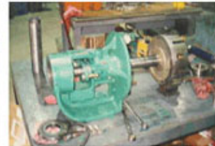
After all the packing is installed, backup rotor from bearing bracket enough to insert the packing gland and the inside bearing cover with the new grease seal. Then push rotor back in bearing bracket.
