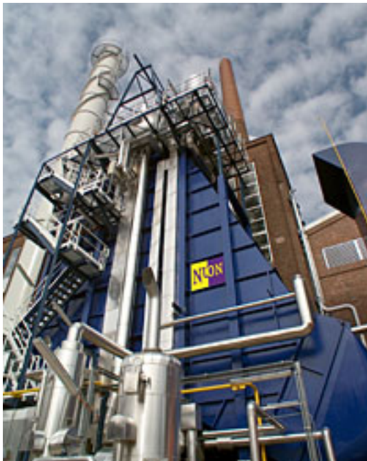
The power station
